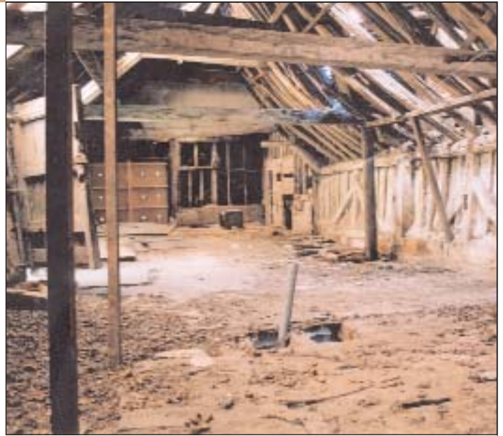
The Malthouse requires urgent conservation work
